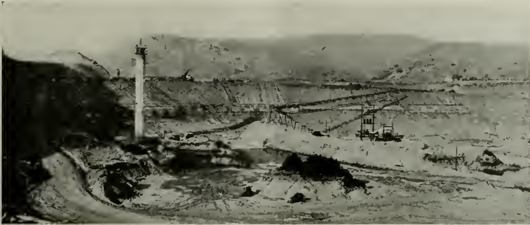
Earth fill dam, contains over 1,100,000 cubic yards of material placed by trucks, tractor-drawn carts and conveyors.
